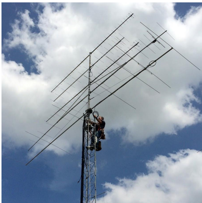
This doesn't look like the "lower" four bands, but George, K5TR, can be seen hard at work getting his VHF/UHF array ready for the contest. From bottom to top (not including George) are seven elements on 50 MHz, 17 elements on 144 MHz, 16 elements on 222 MHz, and a pair of 28-element beams on 432 MHz. [George, K5TR, photo]
